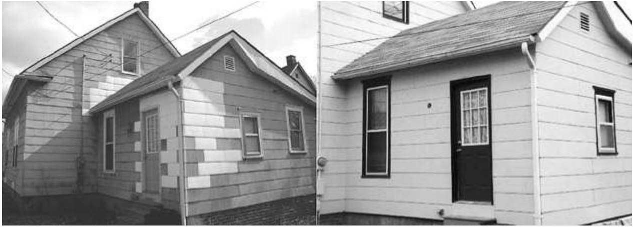
Figure 7. Replacement non-asbestos fiber-cement shingles in place, before being painted and after (photo by author).
