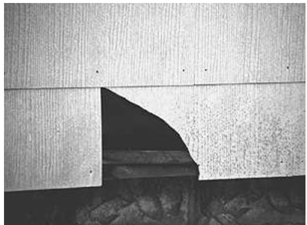
Figure 6. Asbestos-cement products most commonly deteriorate by cracking and chipping. These kinds of deterioration are not typically feasible to repair, and therefore it is recommended that a non-asbestos fiber cement piece be used as a replacement (photo by author).
